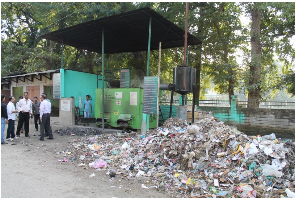
Figure 5-2 Swatch Plasma system Installed by Nagaon Municipal Board for Waste Disposal
