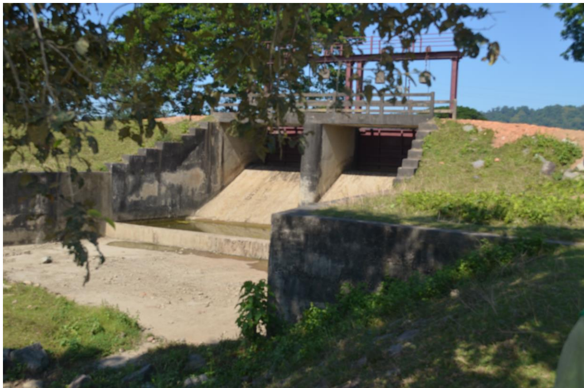
Figure 8-8 Irrigation Canal Regulator at the old course of Kolong (Photo: LBG-DHI Nov 2013)
