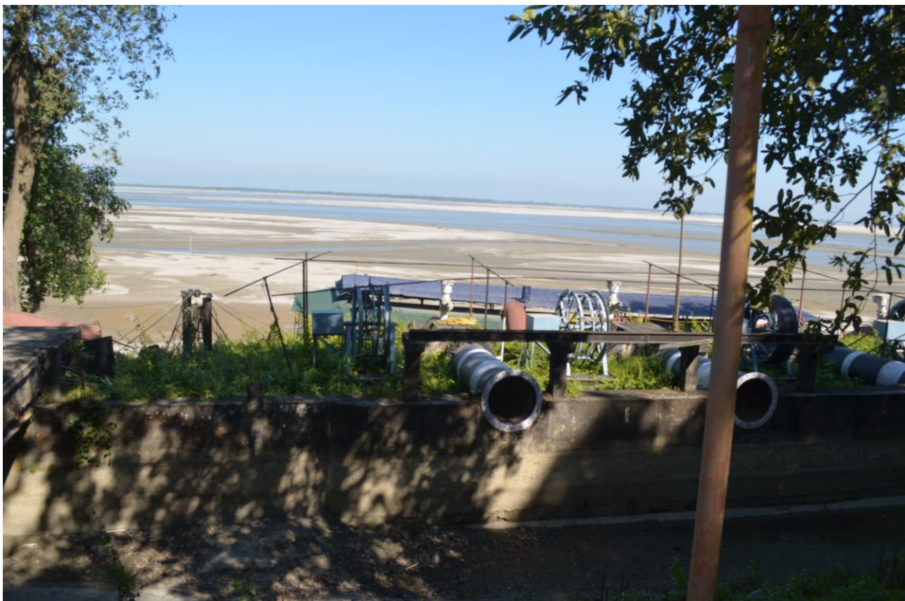
Figure 8-7 Pumps discharging into the Irrigation Canal (Photo: LBG-DHI Nov 2013)
